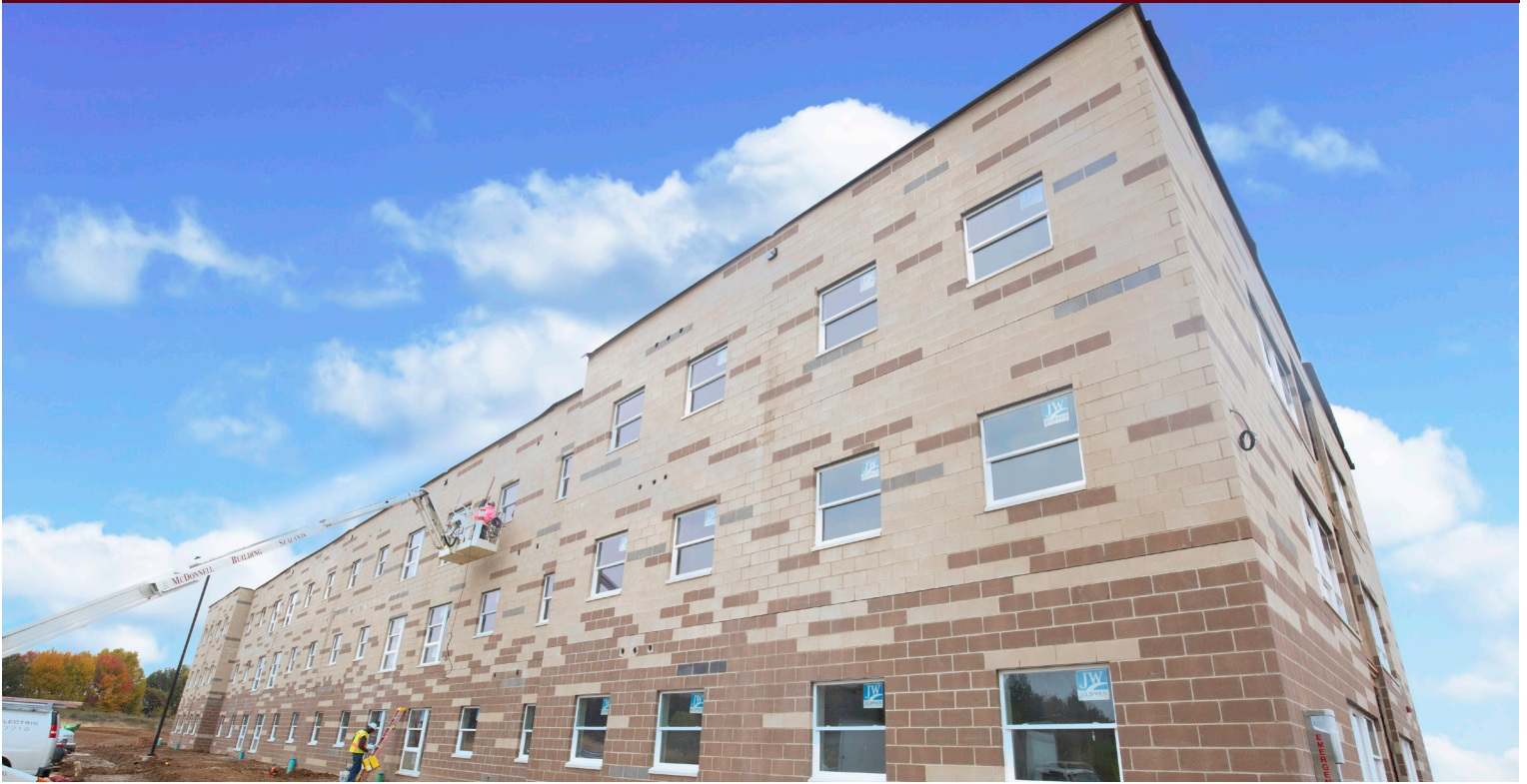
Construction on the Campus Lake Apartments is on schedule. Students are expected to be able to move in after the start of the new year.
